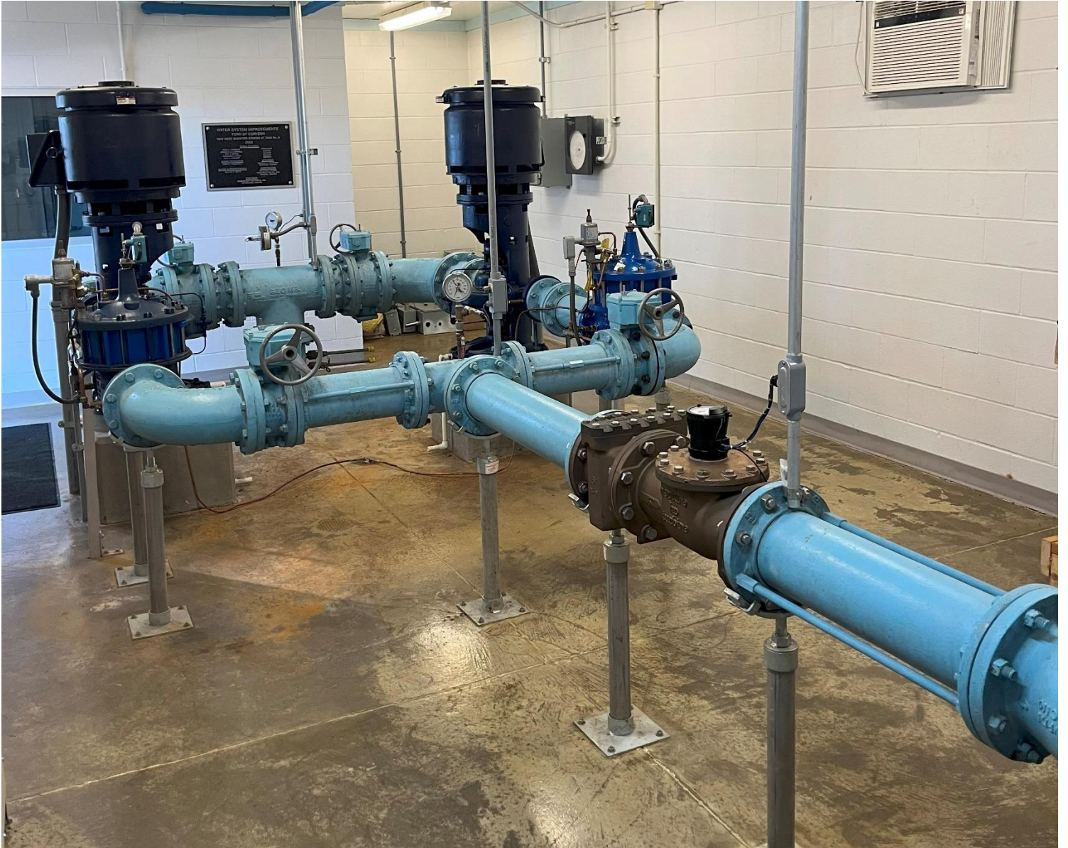
West Booster Interior Showing Two – 1,000 GPM Pumps
