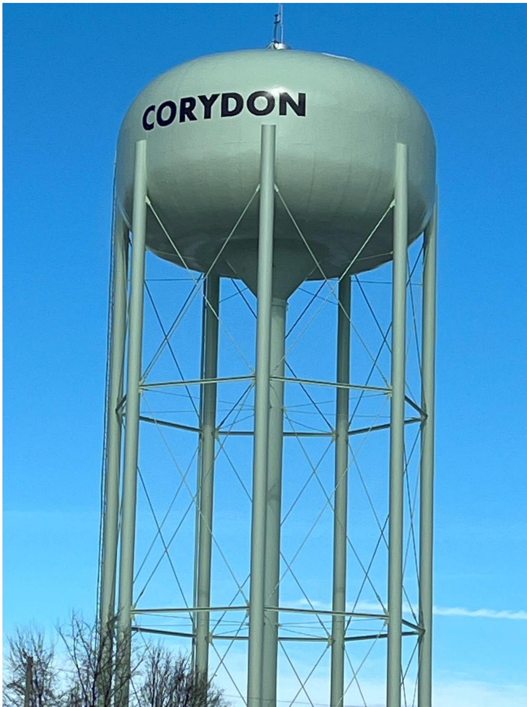
500,000 gallon Industrial Park Storage Tank – Built 1984
