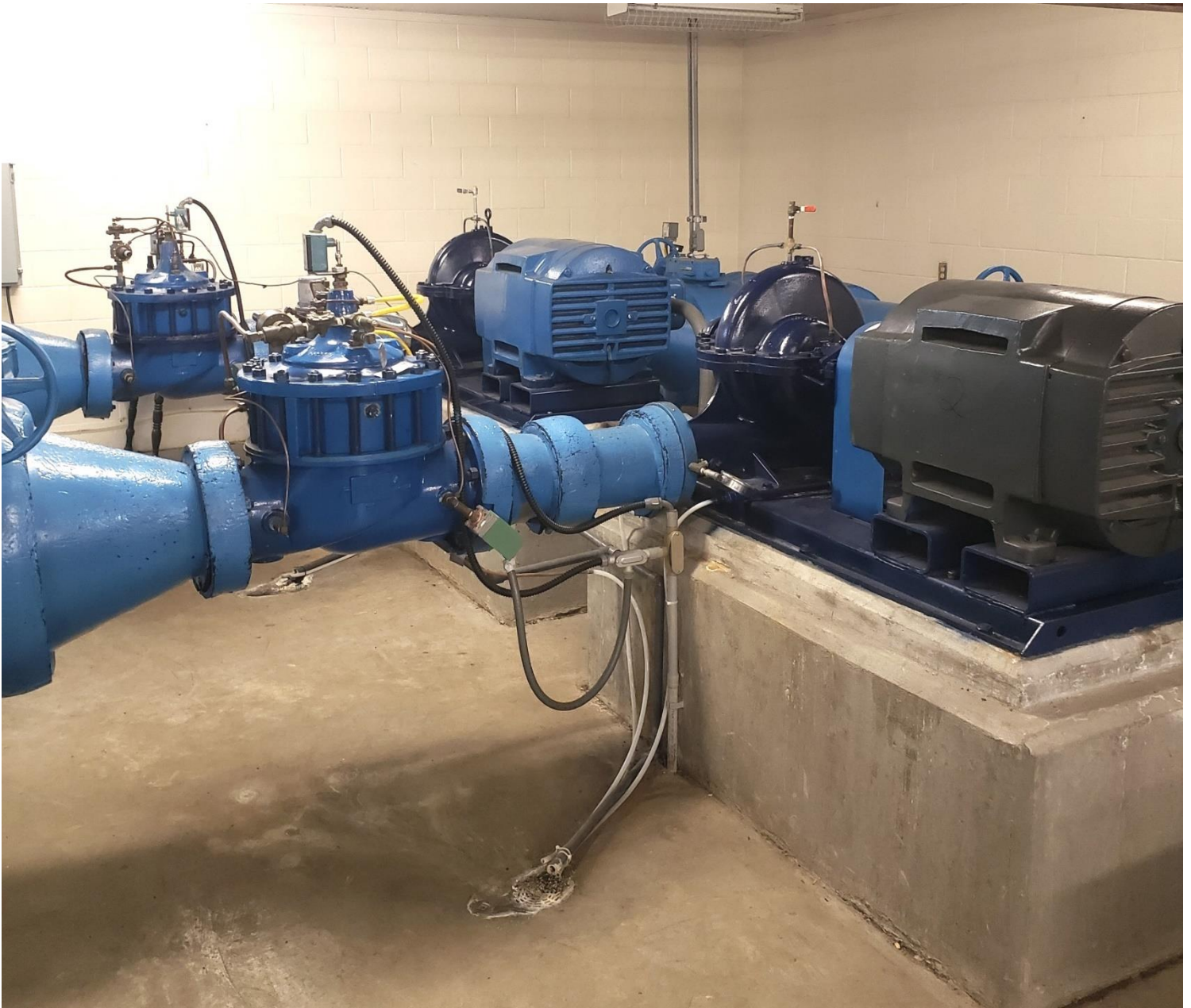
Glidas Booster Station Interior View Showing Two - 2,000 GPM Pumps
